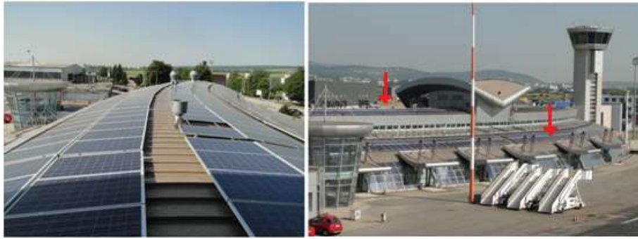
Figure 3 Detail of the photovoltaic panels at the Košice Airport
