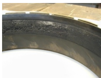
Figure 13 Burnt-out sealing compound in the gas turbine casing above the rotor blades
