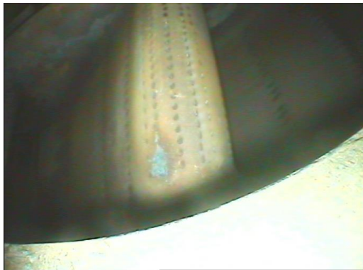
Fig. 4 Gas corrosion on the guiding mechanism of the high-pressure gas turbine (photo Martin Schmidt)
