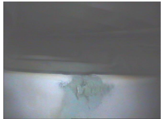
Fig. 5 Material cutting (burn-out) of material on the guide-vanes in the guiding duct of the low pressure turbine of the RD-33 engine (photo Martin Schmidt)
